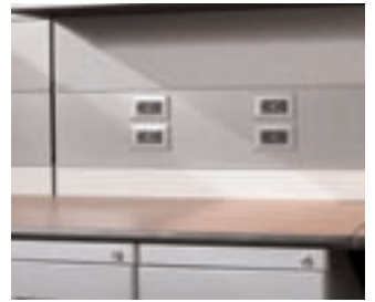
Quad power tile above work surface height.
