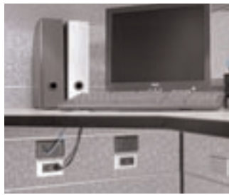
Quad power and data tile below the worksurface
